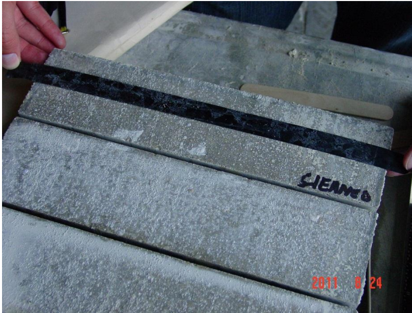
Figure 13. Electrical tape test result on cleaned joint.
