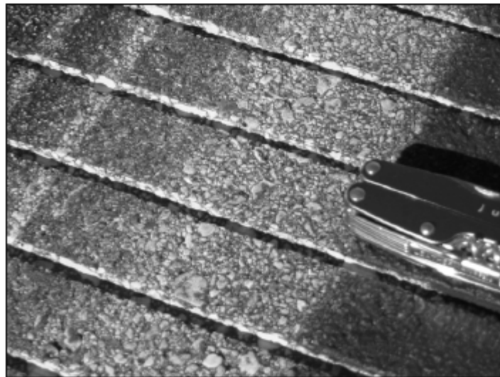
Figure 2 Five-year old saw-cut grooves at Volk Field Air National Guard Base in Wisconsin; the HMA runway regularly supports heavy cargo planes (4)
