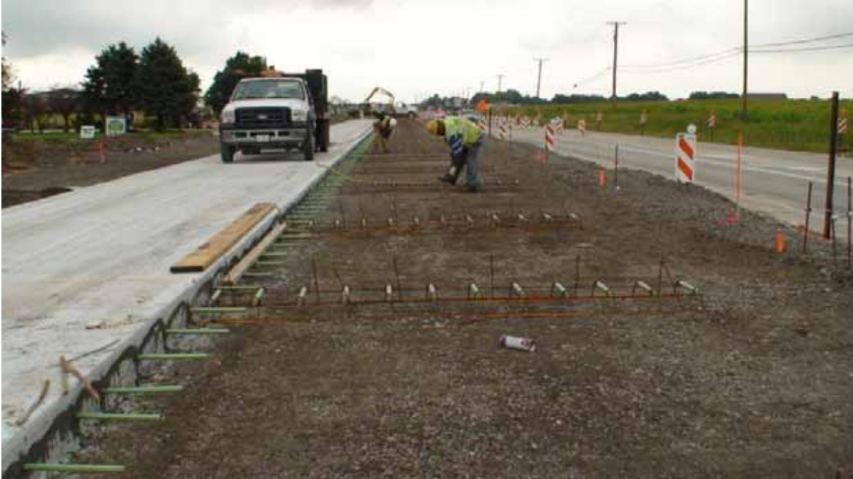
Figure 2 Dowel Basket Placement in High Speed Lane Alongside Recently Poured 9 ¾" Thick Travel Lane
