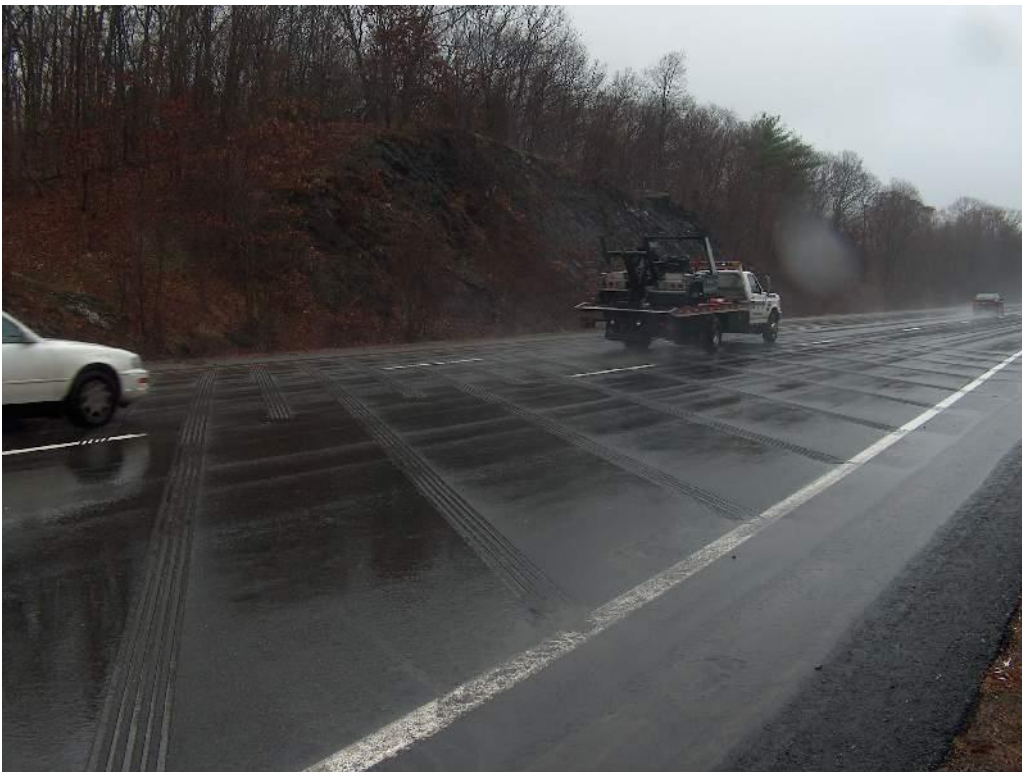
Figure 6 – Grooved Pavement – Moderately Heavy Rain Event (reduced misting behind tires)
