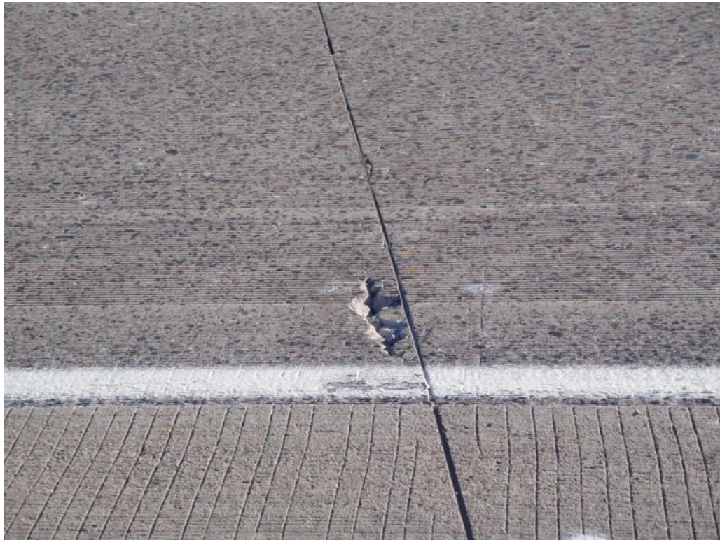
Figure 4-1 Spalling at Joint
