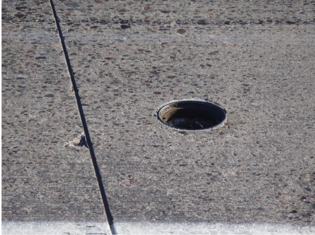
Figure 3-1 Hand Hole in Test Area
