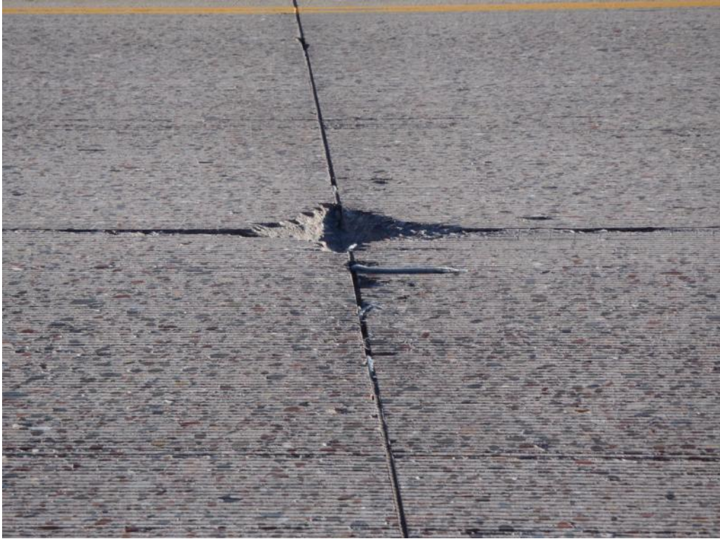
Figure 2-5 Spalling and Backer Rod Failure
