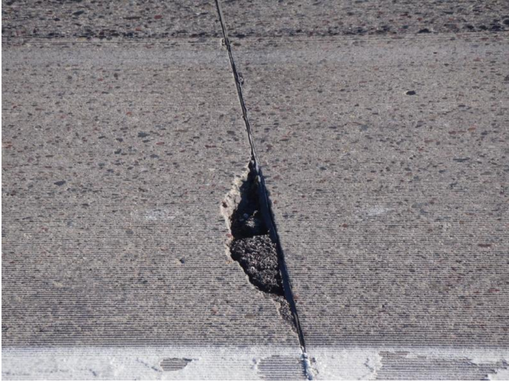
Figure 3-3 Spalled Joint and Failed Repair
