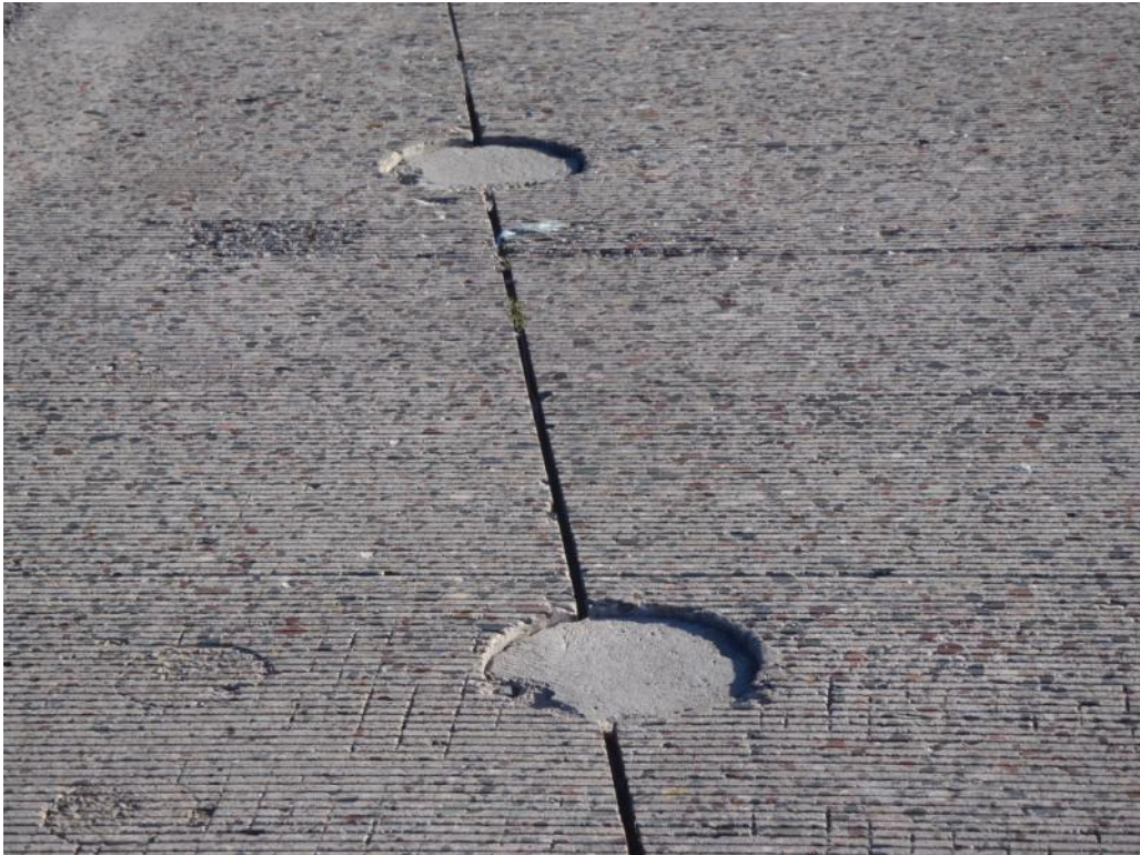
Figure 2-2 Depressed 12 inch Core Hole Repairs and Existing Transverse Tining
