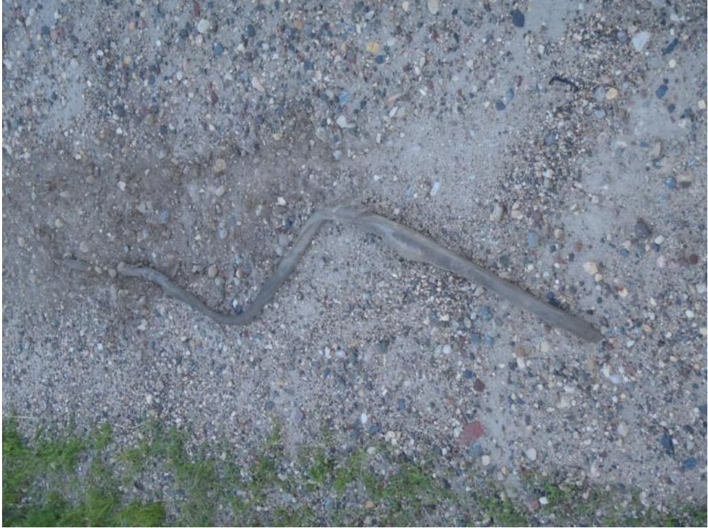
Figure 5-2 Failed Sealant on Shoulder of Roadway
