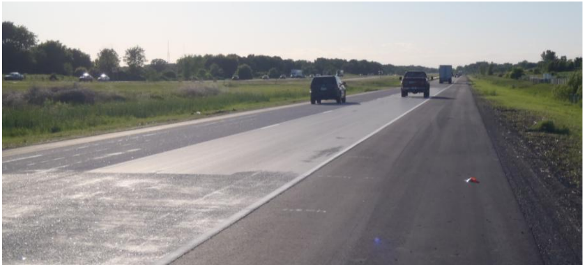
Figure 1-6 NGCS (Travel Lane) and CDG (High Speed Lane) Ground Into Exposed Aggregate Test Section
