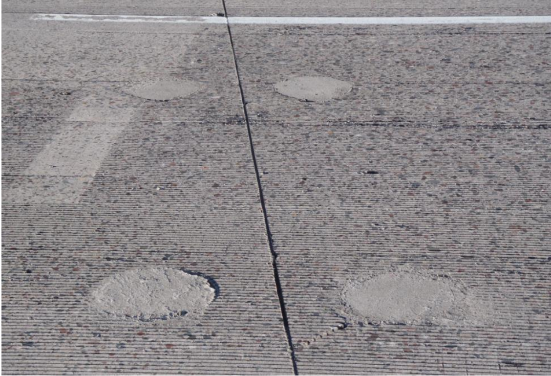
Figure 2-3 12" Core Holes with Good Patches
