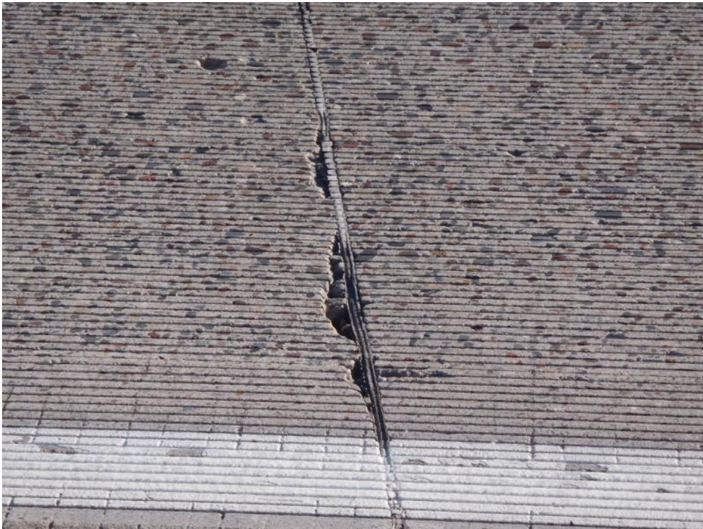
Figure 2-1 Spalling in NGCS LITE Texture (Cell 9)
