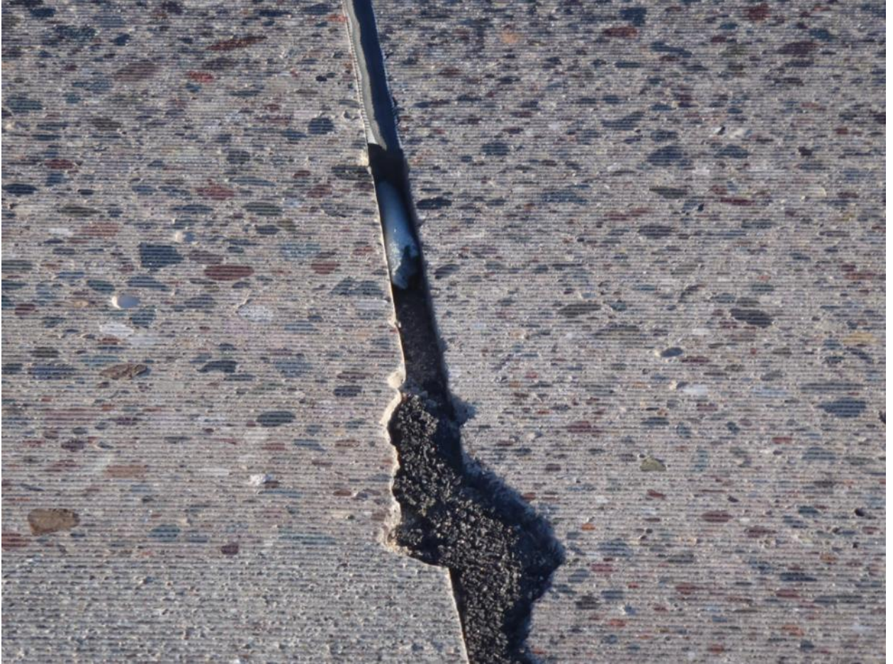
Figure 5-1 Spalled Joint and Failed Sealant in Wide Joint
