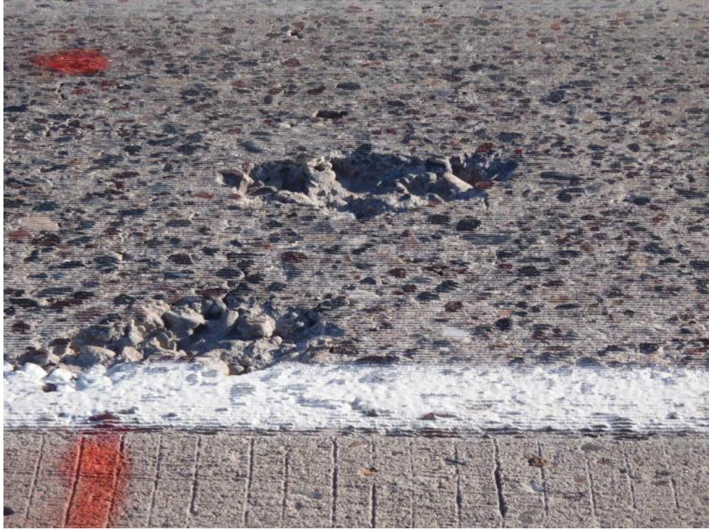
Figure 3-7 Spalls on Surface of Roadway
