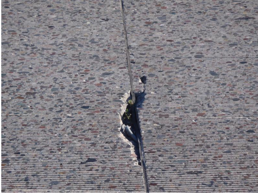
Figure 4-5 Spalling at Joint
