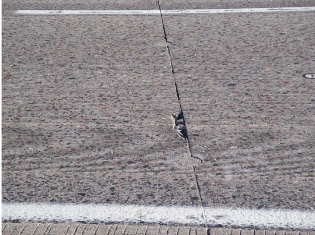
Figure 4-3 6" Core Hole Repairs and Spalling at Joint
