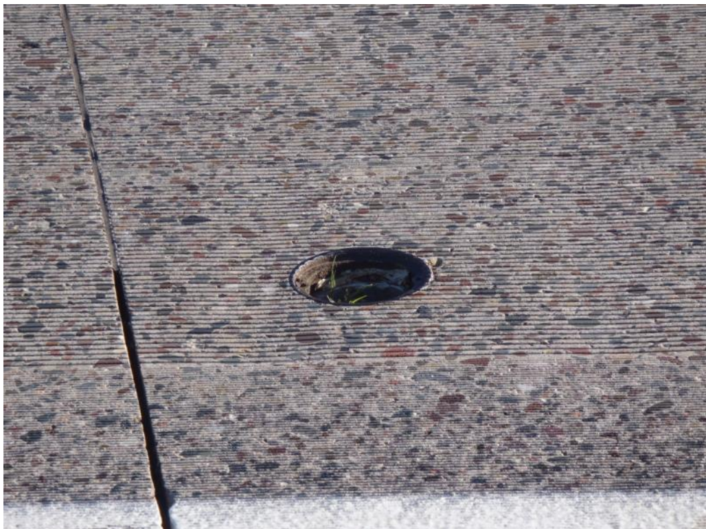
Figure 4-2 Hand Hole with Grass and Sealant Failure in Transverse Joint
