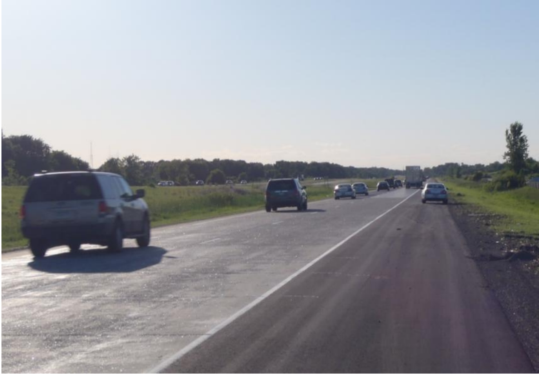
Figure 1-5 NGCS (Shiny Surface) and CDG Section at End of Exposed Aggregate Section
