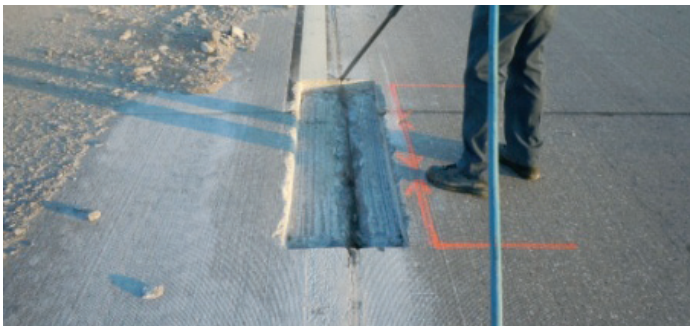
Figure 27. Excess chipping from mill
