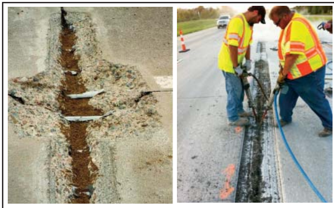
Figure 60. Poor candidate for partial-depth repair (too much sand used, which shortens life)
