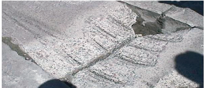
Figure 17. Dish-shaped milling perpendicular to the joint or crack
