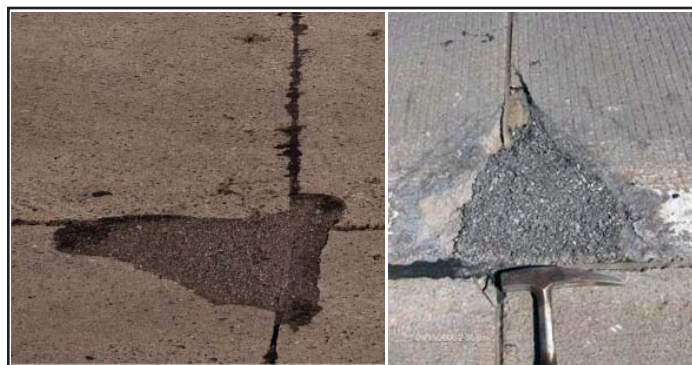
Figure 11. Candidates for Type 3 bottom-half corner joint repair
