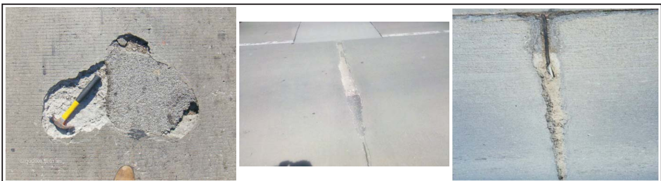
Figure 6. Type 1 spot repair candidates; left to right: spalling, crack, joint
