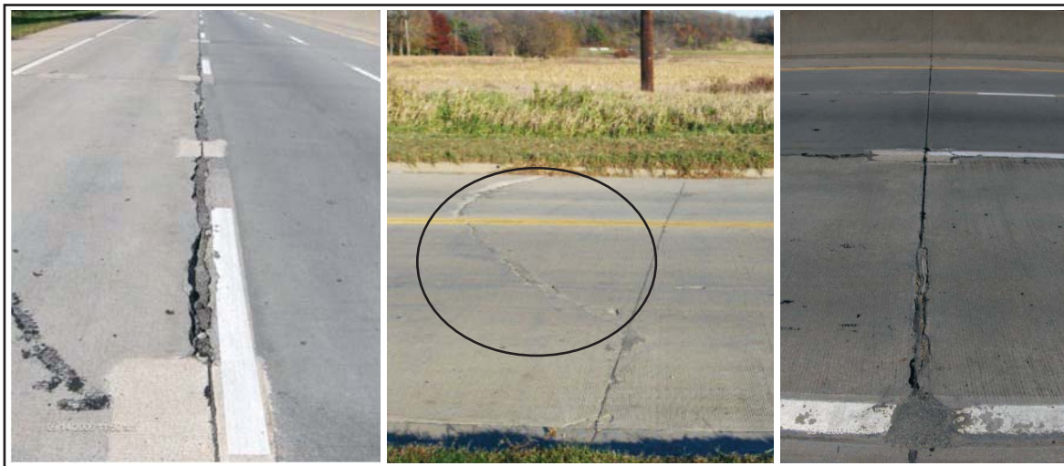
Figure 9. Candidates for Type 2 extended-length repair; left to right: longitudinal joint, transverse crack, transverse joint
