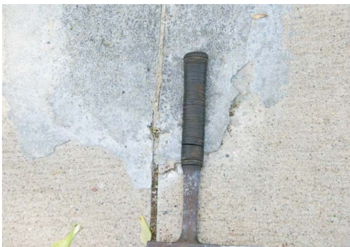
Figure 63. Compression relief failure of (Type 1) partial-depth crack repair on a city street
