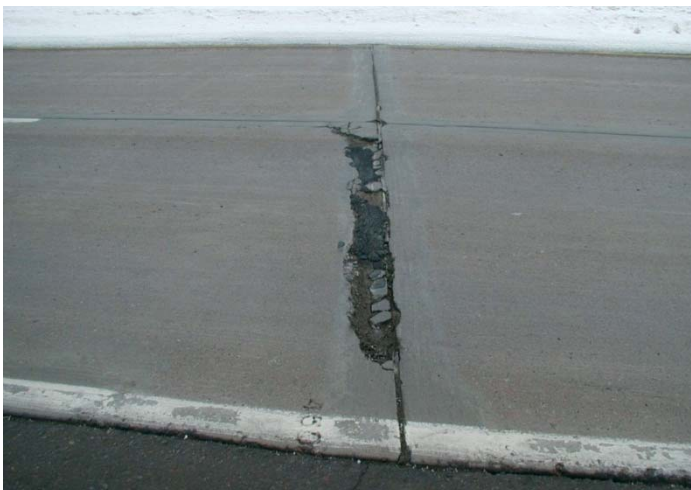
Figure 61. Failed Type 2A repair on an Interstate highway
