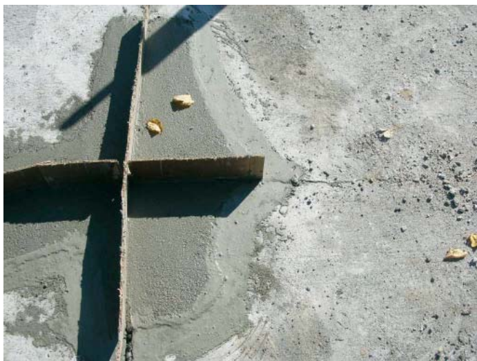
Figure 62. Repair failure because the compression relief material did not extend to end of repair area
