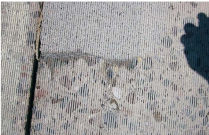
Figure 66. Close up of debonded area at end of a Type 2A partial-depth repair
