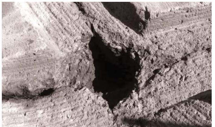
Figure 38. View of hole exposed at intersection of a joint and a crack
