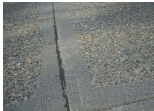
Figure 2. Close-up of partial-depth repair in Hopkins, MN, constructed in 1991 (photo taken 2011)
