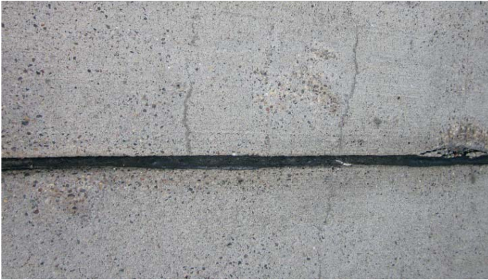
Figure 64. Shrinkage cracks in partial-depth repair
