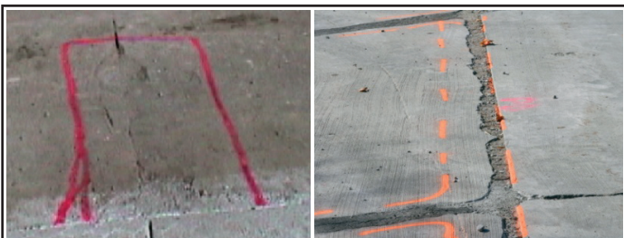
Figure 14. Deteriorated pavement marked for sawing
