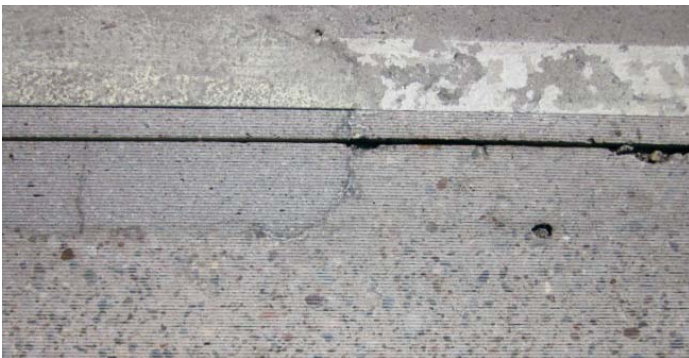
Figure 65. Debonding of patch at end of Type 2 repair
