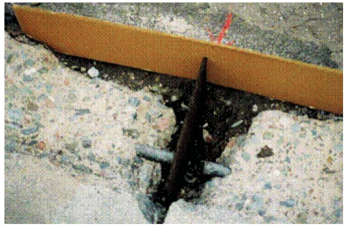
Figure 58. Typical full-depth deterioration at edge of transverse joint
