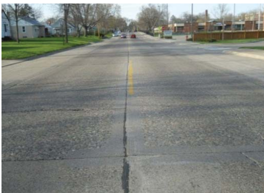
Figure 1. 20-year-old longitudinal and transverse partial-depth repairs in Hopkins, MN (photo taken 2011)
