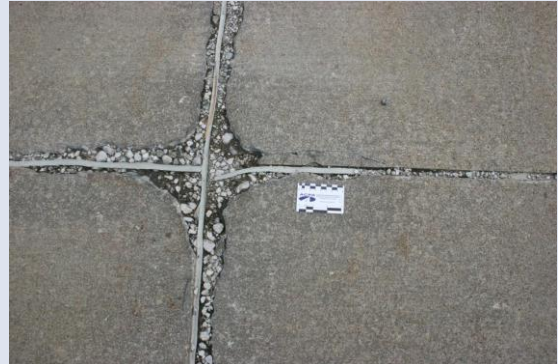
Figure 1 Joint Associated Distress in Parking Area
