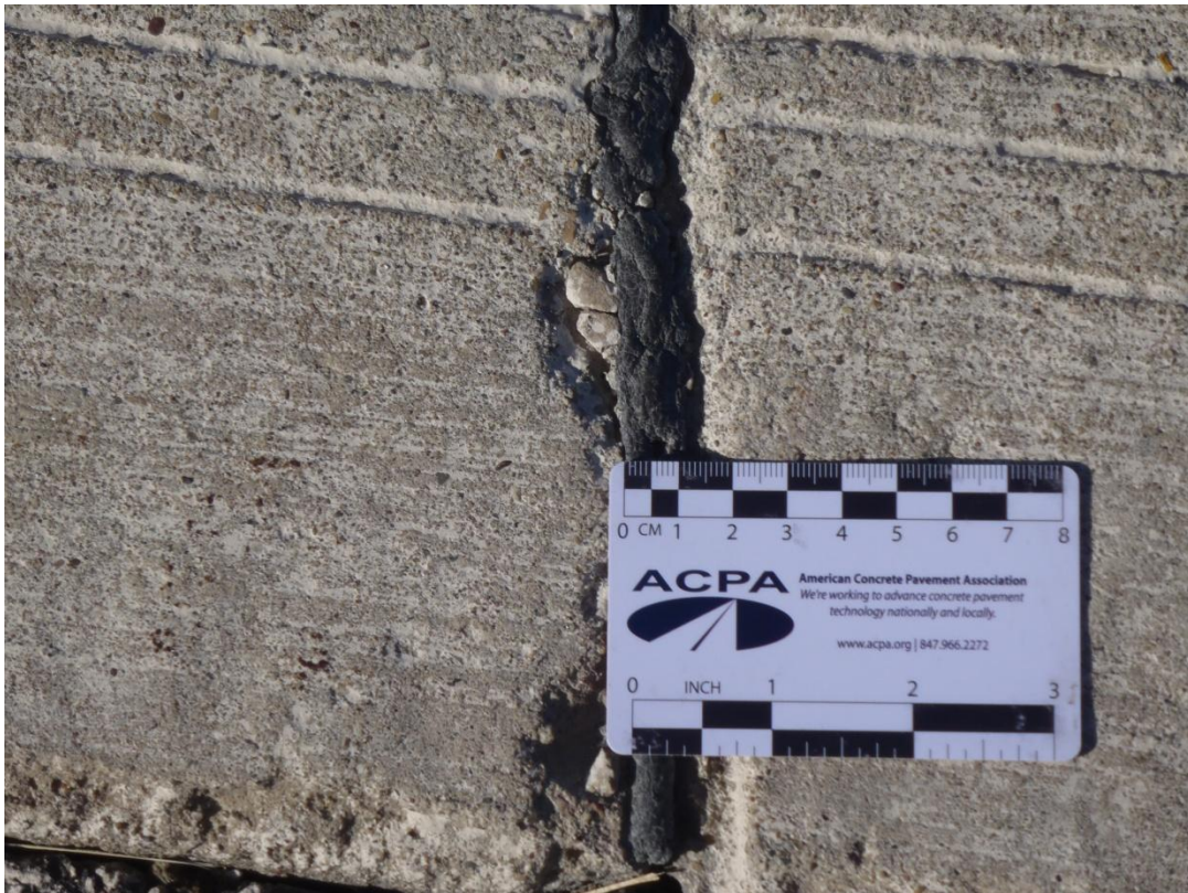
Figure 4-2 Photo of Transverse Joint Sealant Condition and Width
