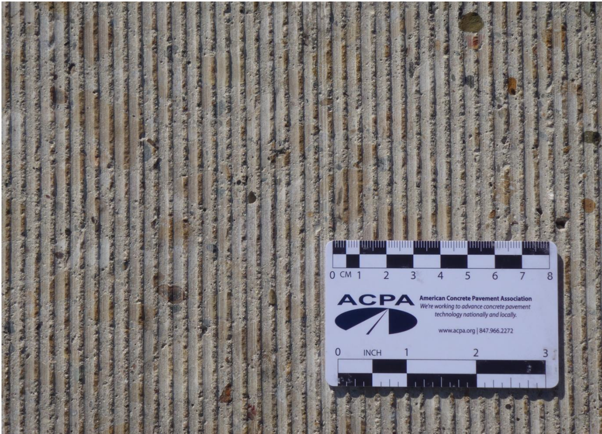
Figure 3-4 Close Up of CDG Texture in Section 3
