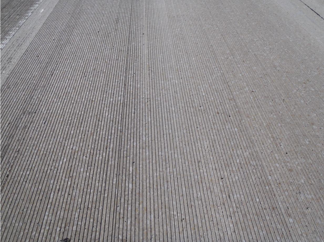
Figure 1-3 View of Flush Ground and Grooved Texture Across Lane in Test Section 1
