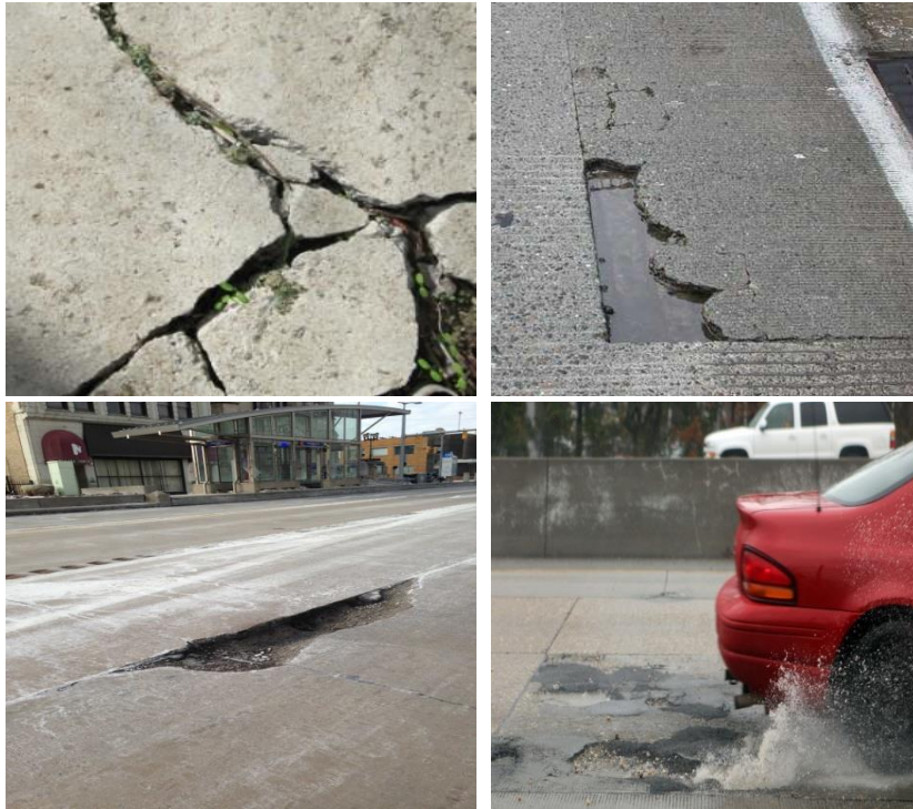
Figure 30 Water Related Damages; Potholes, Corner breaking and Wide Cracks.
